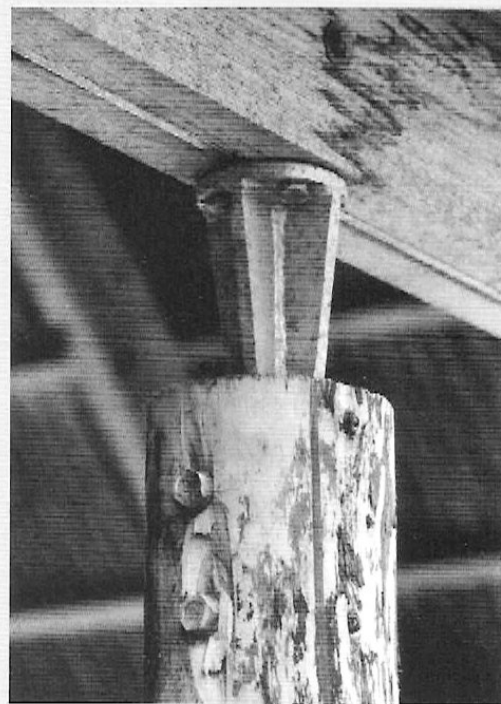
The timber sections of the covered entrance area are bolted or screwed to facilitate their dismantling.
